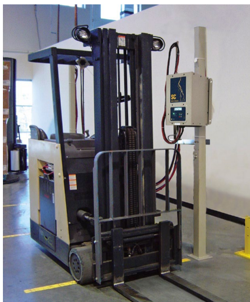
A typical model SC charger installation
