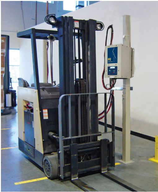
A typical model FC charger installation
